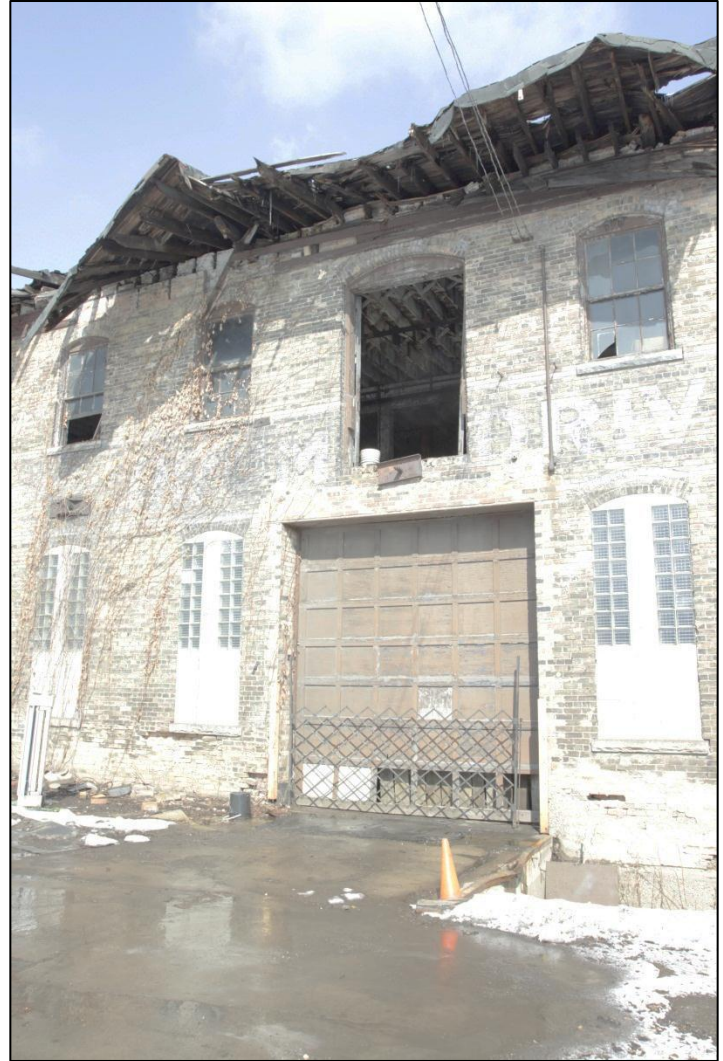
An overhead garage door on the south wall is a non-historic alteration. Several original windows on the second floor have broken glass and all of the window openings on the first floor have been filled with concrete and glass blocks.
