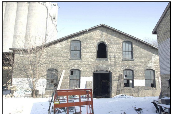
These 2013 photographs illustrate the foundry's structural and material decay.
